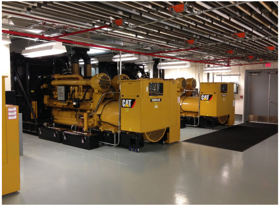
Figure 1. Generator sets housed in the data center facility. Each of the four generator sets is rated for 2 MW and is powered by a CAT 3516 engine.
